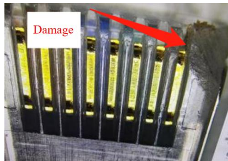
Figure 5-23 Damage of RJ45 connector without dust cap
